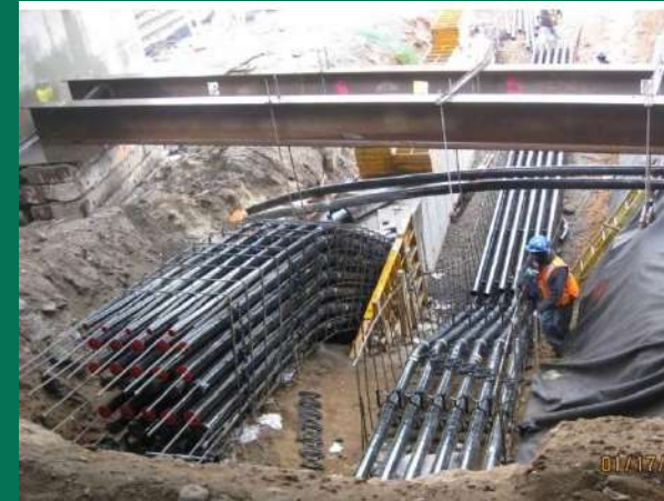
Oil-Static line (high voltage power line cooled by oil)
